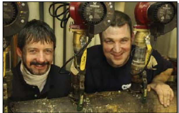
Kevin Amyot of H.A. Manosh Corp. (left) with installer Ed Friedrich of County Plumbing & Heating in Morrisville, Vermont: "Ed is highly experienced," says Amyot, "one of the best boiler people in the area, in our opinion."
