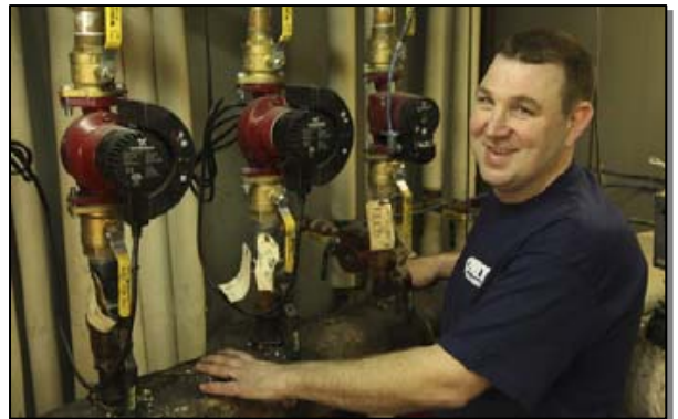
Installer Ed Friedrich with two of the MAGNA units and the one ALPHA unit he installed at Sunset: "I set all four circulators on AutoAdapt," says Friedrich, "because I knew that the load-matching feature along with the design of the motor itself would deliver the major reductions in electrical consumption."
