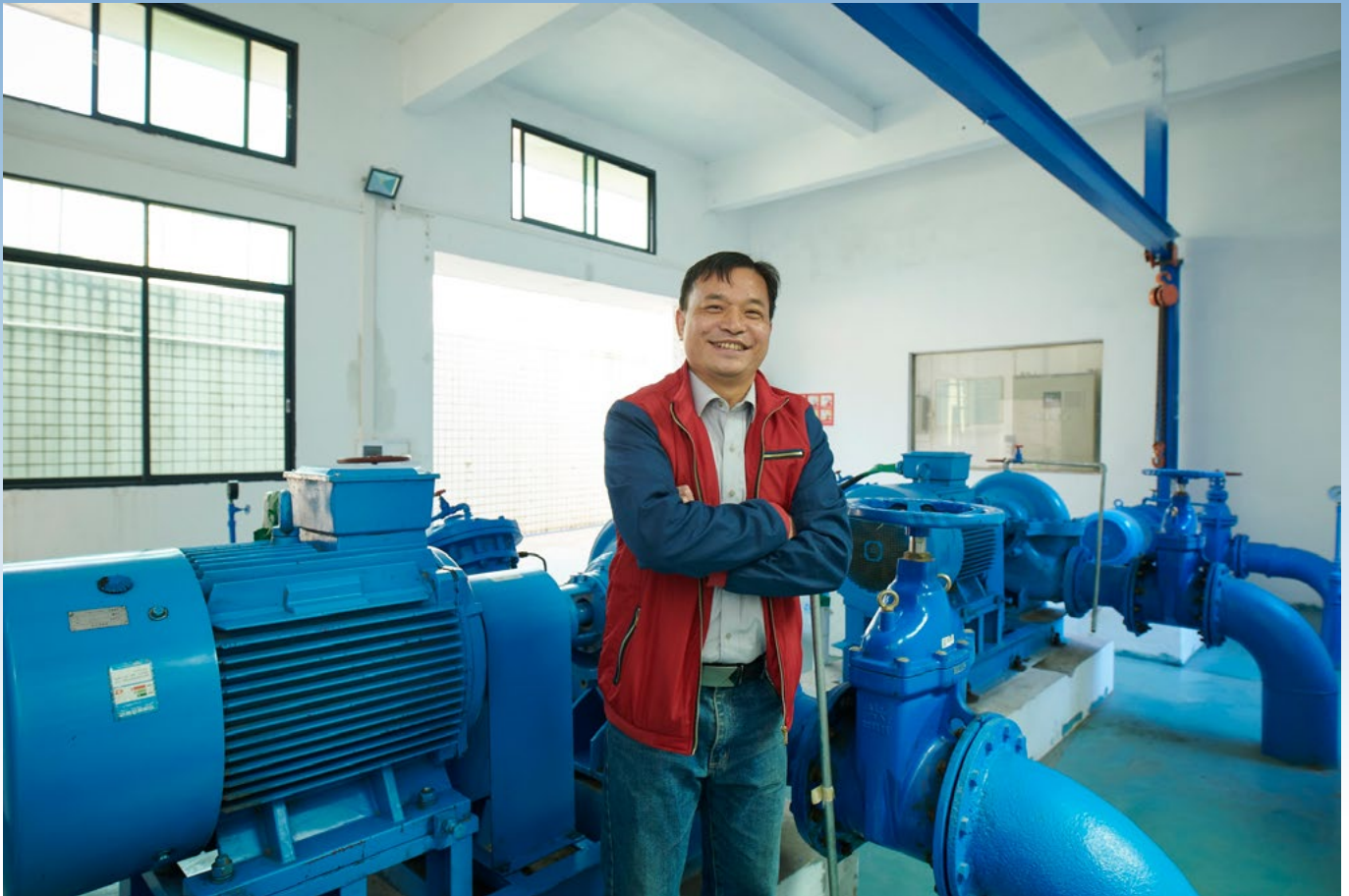
Zhong Jinshou, Head of Department at Qujiang District Water Supply Management, says he enjoys the stability and quieter operation of the new Grundfos pumps.
