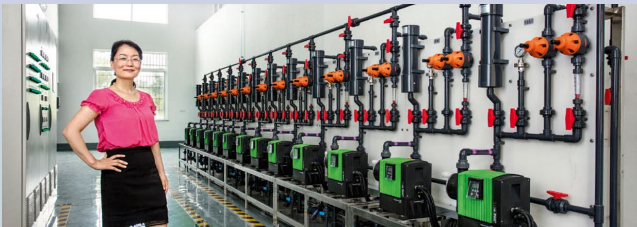
"These pumps ensure the water safety of 1.5 million citizens. From my side, it is an important issue with great social value," says Jiang Yarong, General Manager, Hangzhou Jijie Environment Protection Technology Company.
