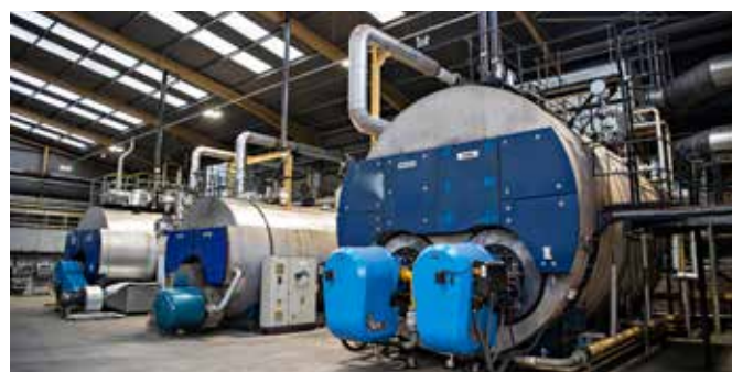
Three of the steam boilers at the William Grant & Sons’ Girvan Distillery in Scotland.
