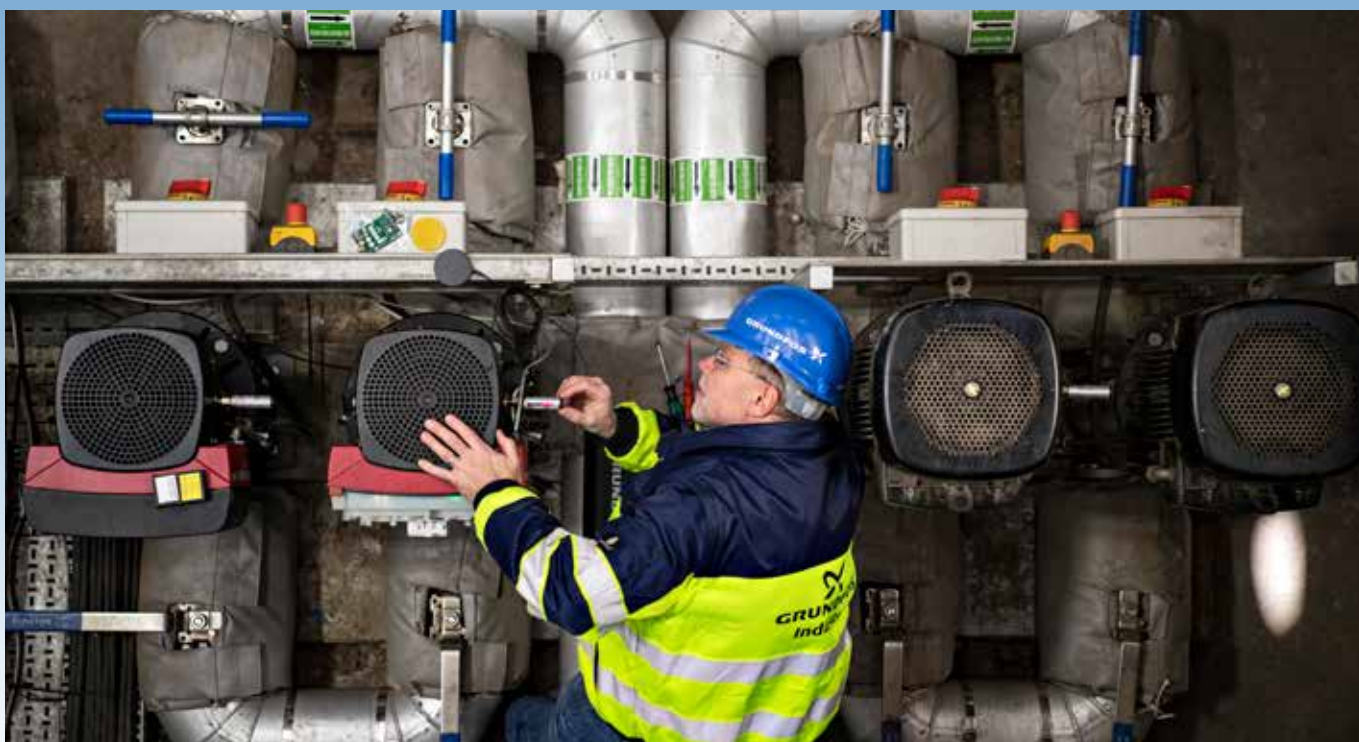
Grundfos Senior Application Manager Michael Rasmussen at one of the new CRIE pumps for the boiler feed level control at Grant's.
