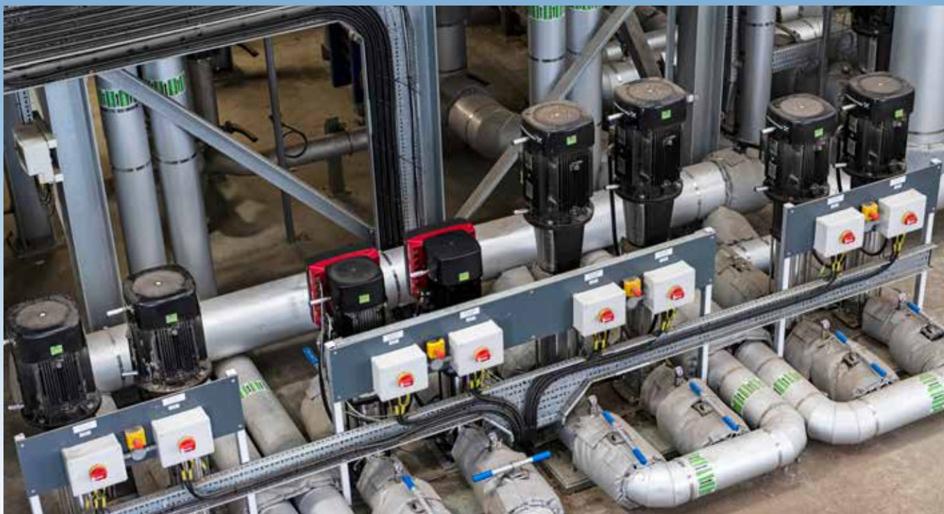
The Grundfos CRIE pumps (with red cover just left of centre) have built-in variable speed drives. These replace the usual modulating valves from the boiler feed control system. The pumps go up and down in speed, depending on demand.
