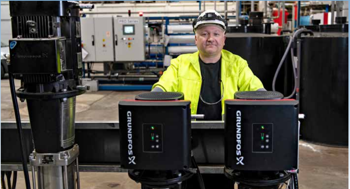
Grant's Maintenance Leader Scott Curran at the new Grundfos CRE pumps, adjacent to the traditional fixed speed pumps that are typically connected to boiler feed.
