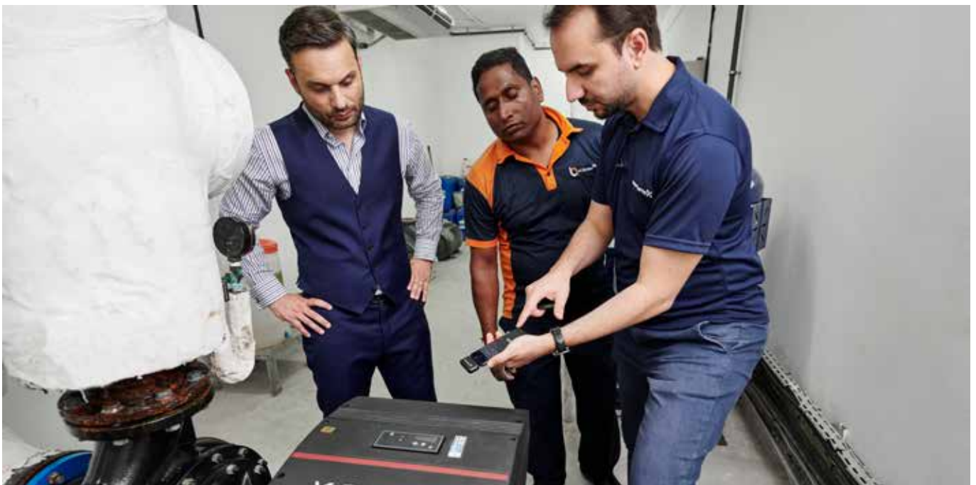
Vasileios Vatisas of H&H (left) and Indigo Tower’s Facility Manager learn how to monitor the Grundfos NBE pumps via a smartphone Grundfos GO app from a Grundfos Service technician (right).
