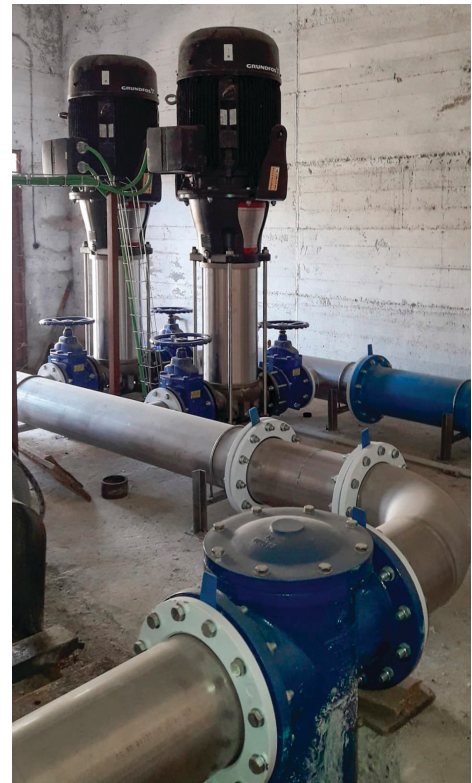
Two Grundfos CRN pumps provide a reliable water supply to thousands of people.
