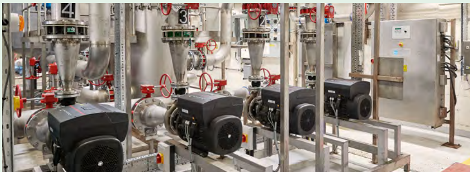
The Grundfos beverage network supply pumps.
