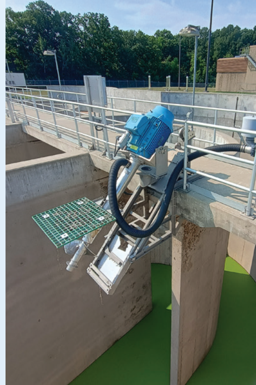
The facility has two oxidation ditches (above), but operates only one at a time, allowing the second ditch (right) to remain offline as a backup or for maintenance.
