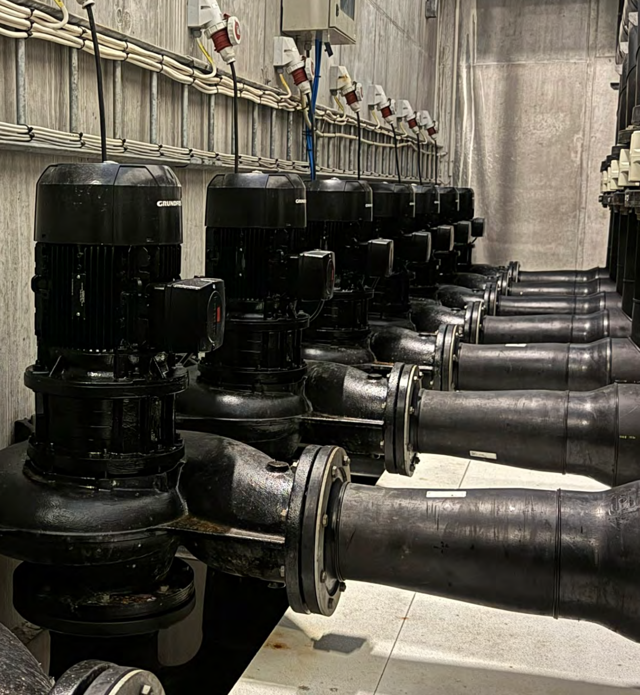
Image: NB Duplex pumps at Lerøy Belsvik, Hellandsjøen, Norway
