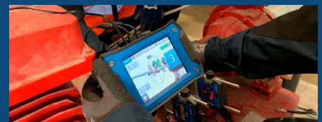
A laser alignment tool helps to make sure the pump motor shaft is in line on the Grundfos fire pumps.
