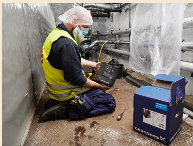
Installing a Grundfos MIXIT at Envases in Odense, Denmark.
