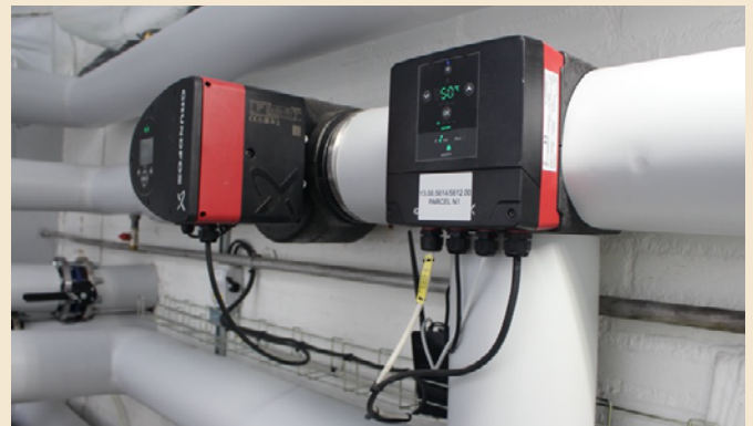
Image: The mixing loop after the MIXIT retrofit. The Grundfos MIXIT unit is on the right, and a Grundfos MAGNA3 circulation pump is on the left.
