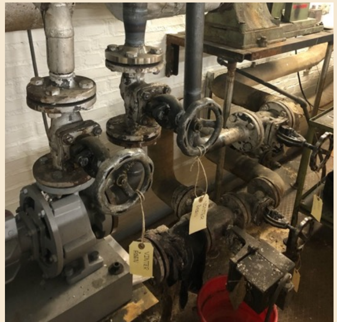
Image: An Envases mixing loop before the MIXIT retrofit.
