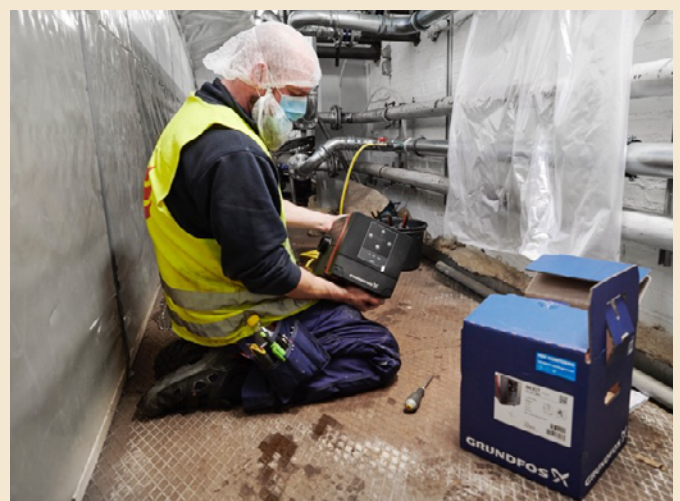
Image: Installing a Grundfos MIXIT at Envases in Odense, Denmark.
