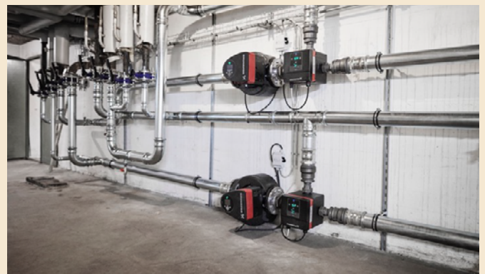
Image: Two freshly installed mixing loops with Grundfos MIXITs and MAGNA3 at Envases.
