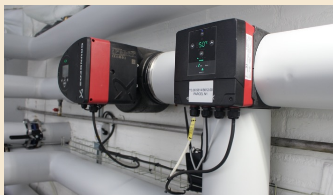
The mixing loop after the MIXIT retrofit. The Grundfos MIXIT unit is on the right, and a Grundfos MAGNA3 circulation pump is on the left.
