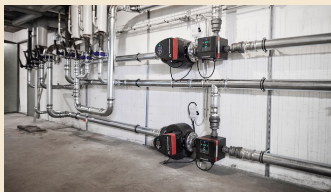
Two freshly installed mixing loops with Grundfos MIXITs and MAGNA3 at Envases.
