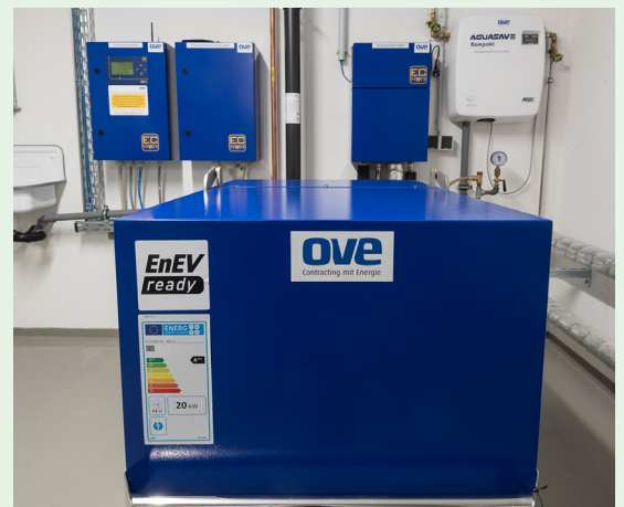
The main heat generator is a compact CHP system with 21 kW of thermal and 9 kW of electrical output.
