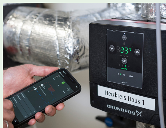
The wireless interface makes it possible to commission and monitor the MIXIT control unit using the Grundfos GO Remote app.
