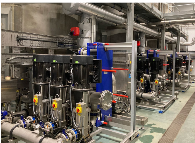
The four Hydro MPC-E pressure booster sets with Grundfos CR pumps.
