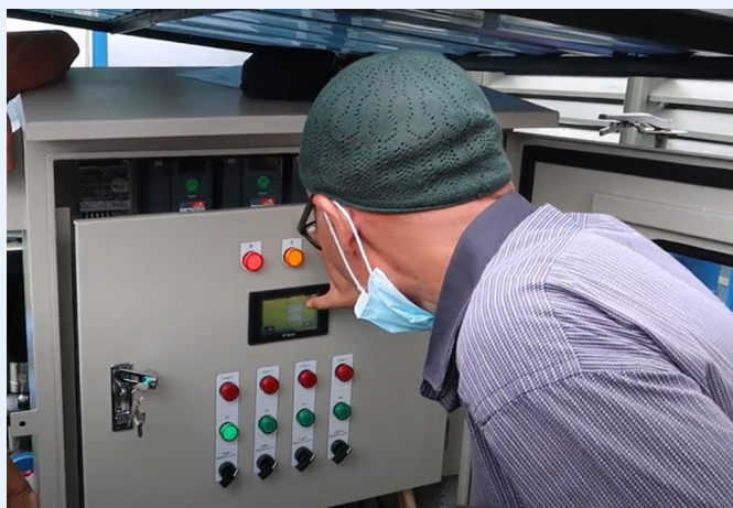
The new control panel
