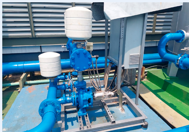
The existing water supply pumps were inefficient and noisy.
