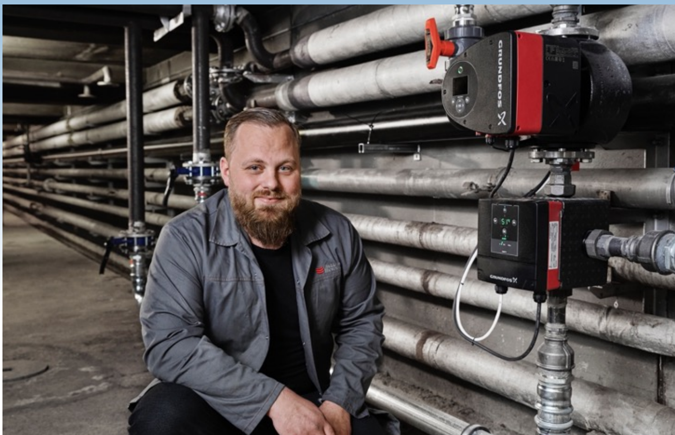
Image: Daniel Bagger, Facility Supervisor at Envases in Odense, Denmark, says, “We can now control our heating system down to the smallest detail.”
