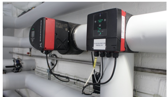
Image: The mixing loop after the MIXIT retrofit. The Grundfos MIXIT unit is on the right, and a Grundfos MAGNA3 circulation pump is on the left.
