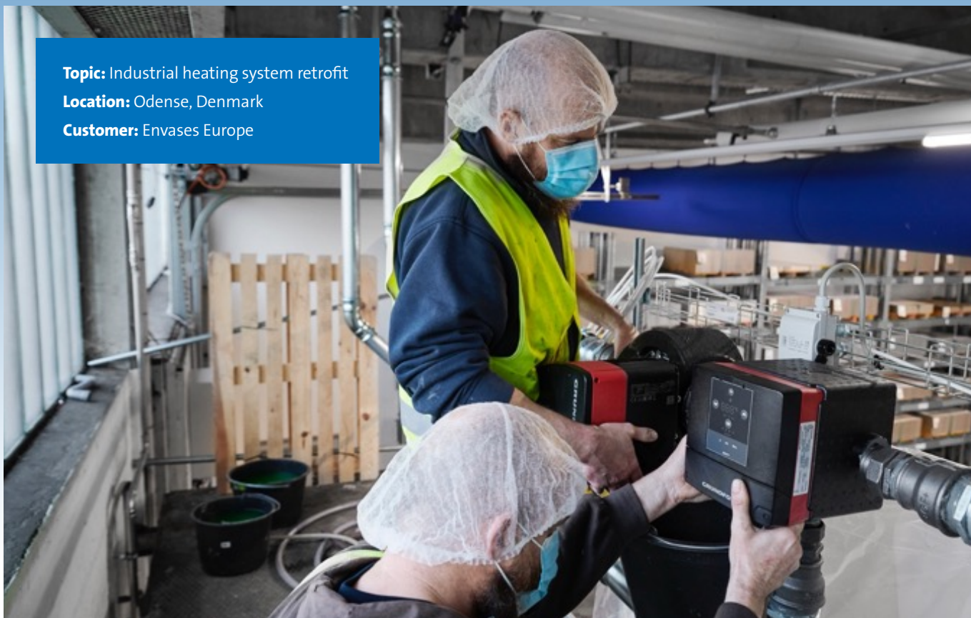
Image: Installing a MIXIT unit by a MAGNA3 circulation pump for the Envas HVAC system.
