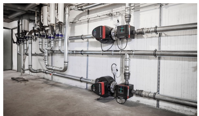
Image: Two freshly installed mixing loops with Grundfos MIXITs and MAGNA3 at Envases.
