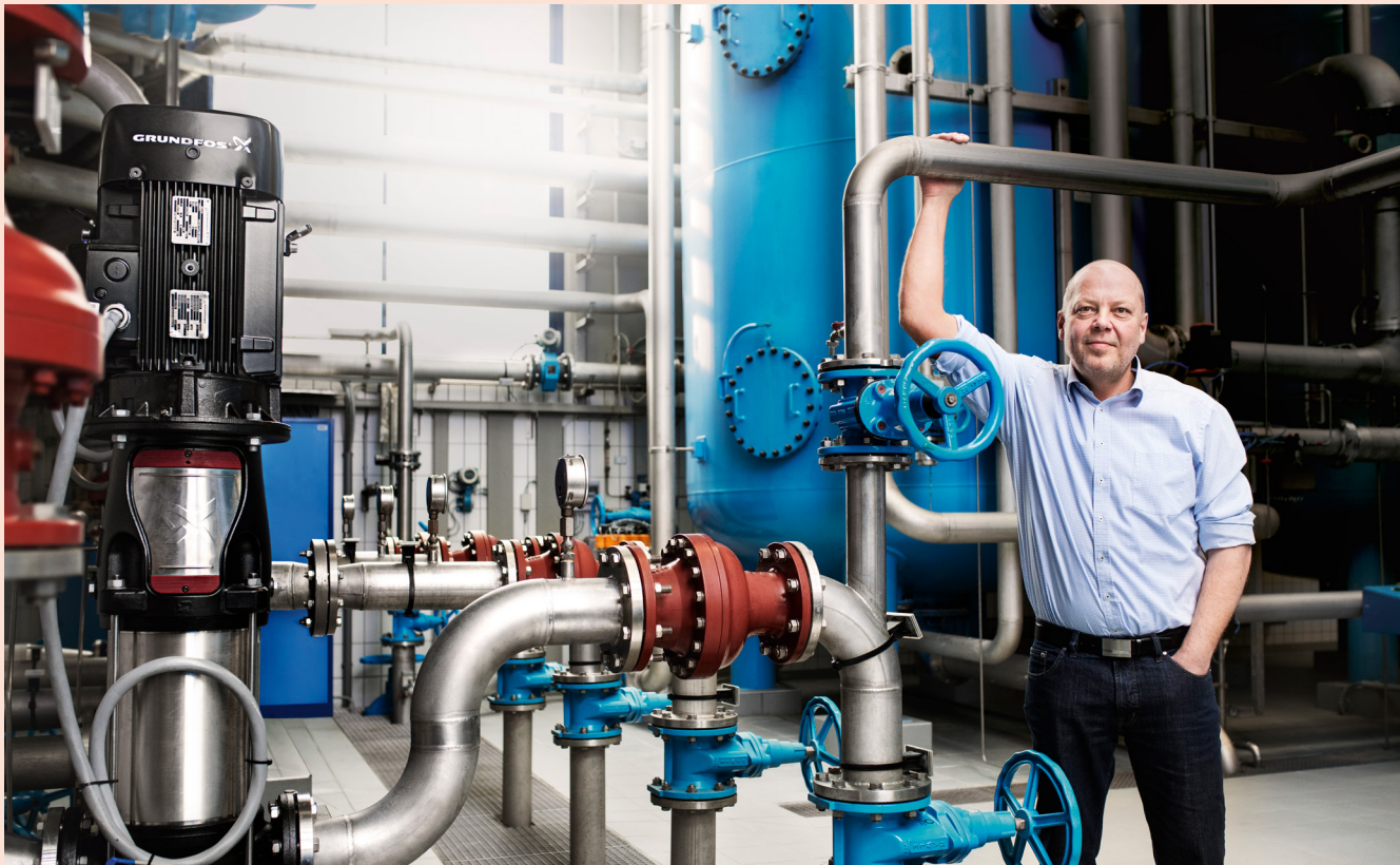
Christian Portschy stands with the Grundfos CR-95 pump for water boosting. Portschy is managing director of Wasserverband Südliches Burgenland (WWSB), the water utility of Southern Burgenland in Oberwart, Austria.
