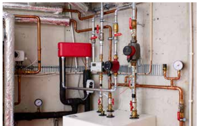
Grundfos has supplied the Urban Rigger with several advanced and energy-efficient products. Besides lifting stations for wastewater and ALPHA2 circulators for water supply, several UNILIFT KP250 secure the rigger against water overflow.
