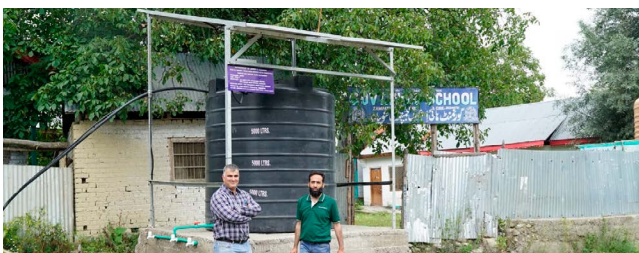
Syed Irfan Bukhari and Zubair Majid of installation partner M/S SIAB Surgiments at one of 36 solar pumping stations at Kasnaad.
