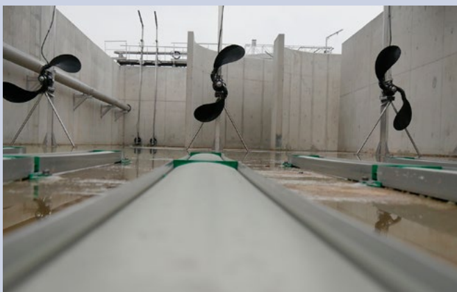
Installation of the Grundfos flowmakers, which helped modernize the wastewater tanks at Tomaszów.
