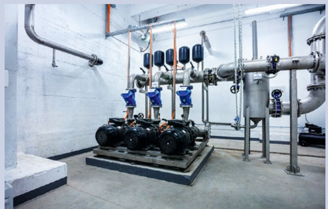
The Tomaszów Mazowiecki plant uses a Grundfos Hydro MPC pressure boosting system for process water. “I buy it from Grundfos for all my projects in Poland,” says Contract Manager Adam Bierut of Cadagua.
