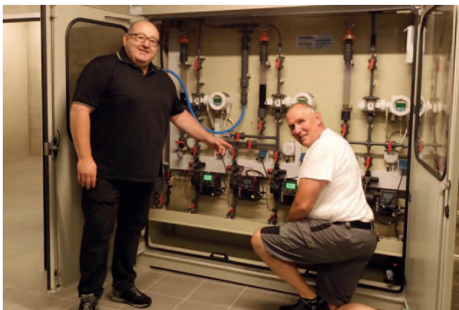
Checking the dosing pumps used. Right: Karl Steck, Operations Manager, left: Maik Wötzel, Sales Representative at Grundfos
