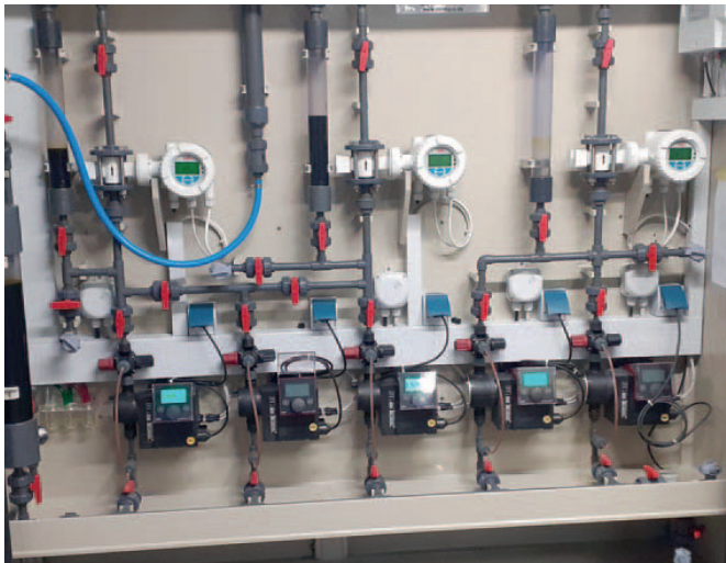
Five DDA 30-4 AR dosing pumps are used to add ferric chloride
