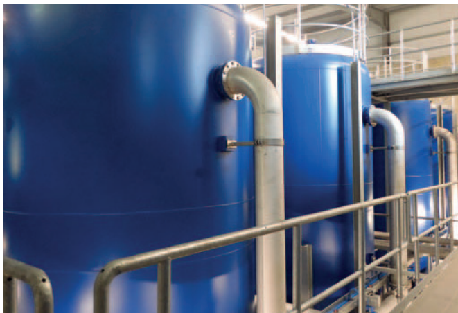
Active carbon filters for the fourth treatment stage arranged in six lines, each with two filter tanks, Q_{max} is 90 l/sec
