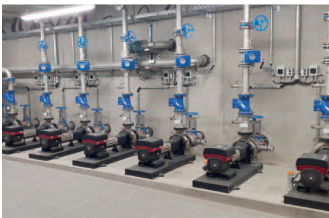
Frequency-controlled standard pumps are used for feeding the sand and coal filters and for backwashing
