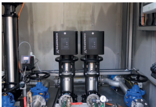
The entire pump system, as well as its control system, is mounted in the container. The system can be used at any time – even at short notice.
