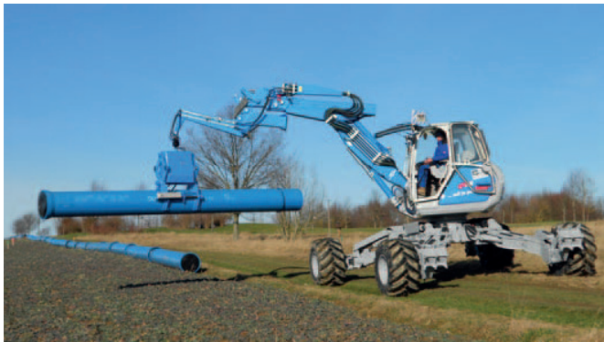
Open-cut pipe laying. A specialist vehicle lays the DN 500 pipes using a process developed by Norbert Schütz.
