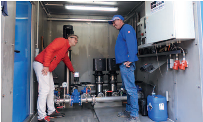
Reviewing operations in the container at the Wemding transfer site. Left: Christopher Filchner, Key Account Manager, Grundfos GmbH, Right: Anton Schütz, Pipe Network Foreman, Senior Site Manager and Managing Director of Norbert Schütz GmbH & Co.KG, Boos, Germany
