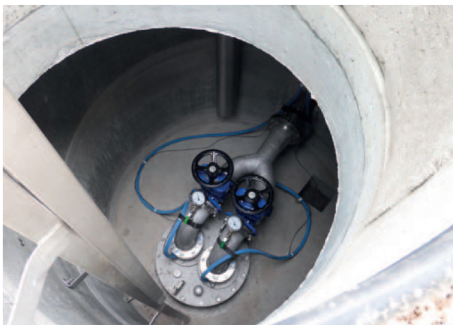
SP borehole pump after installation
