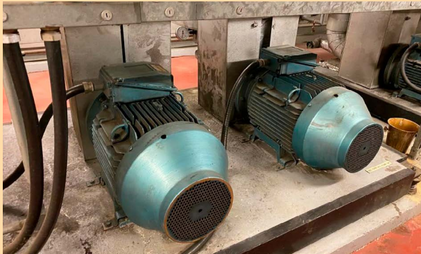
Before and after: Secondary CHW AHU pumps 5 & 6
