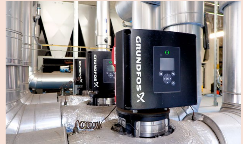
Grundfos TPE pumps for closed loop circulation at the Escaldes-Engordany heating/cooling production site.
