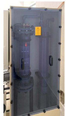
The Grundfos Selcoperm in Sinjar
