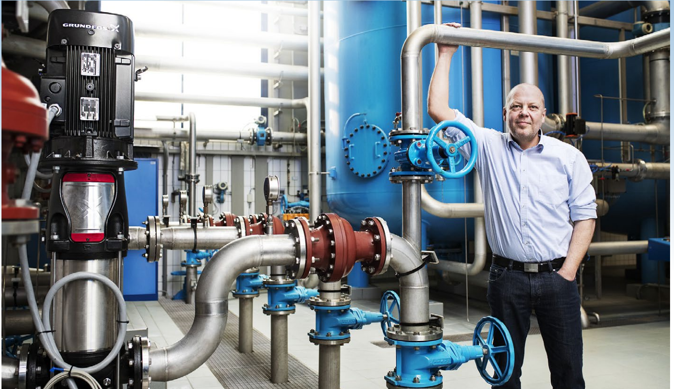
Christian Portschy stands with the Grundfos CR-95 pump for water boosting. Portschy is managing director of Wasserverband Südliches Burgenland (WVSB), the water utility of Southern Burgenland in Oberwart, Austria.
