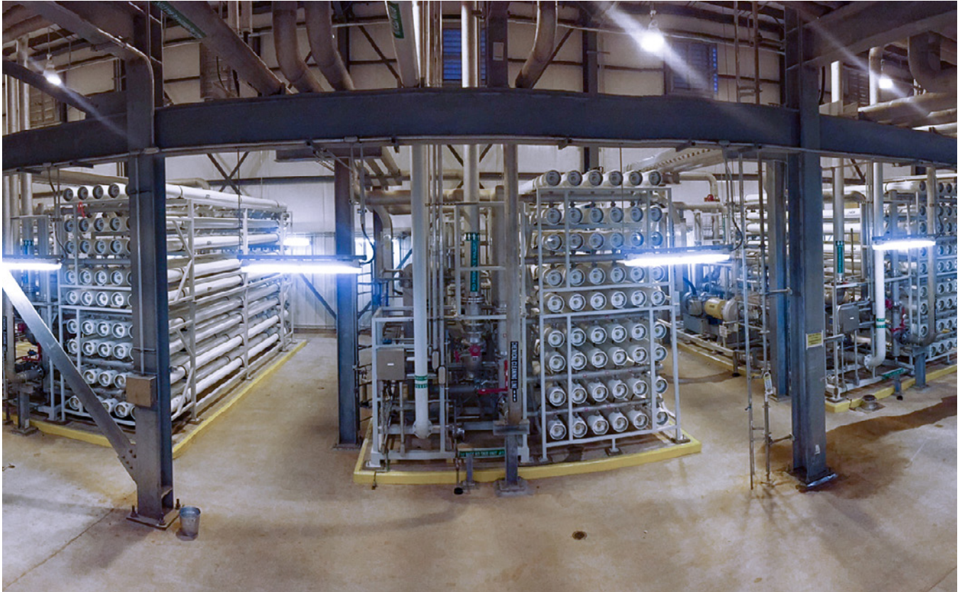
Enid RO Facility
