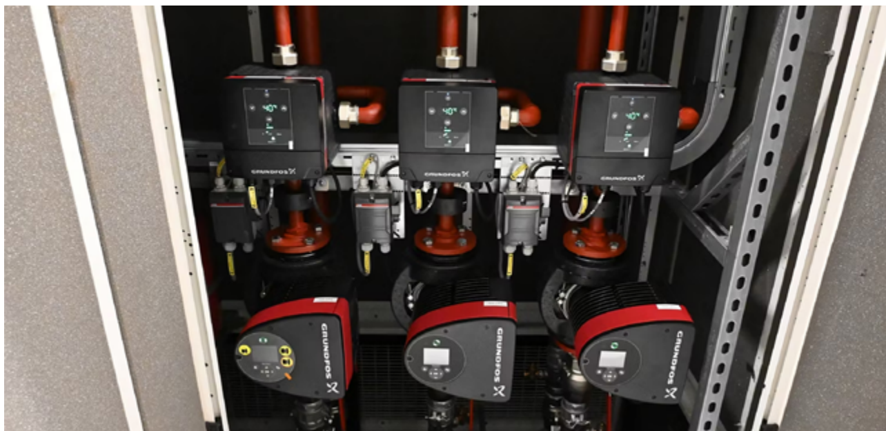
Figure 11 NorthC data centre intelligent flow-control installation
