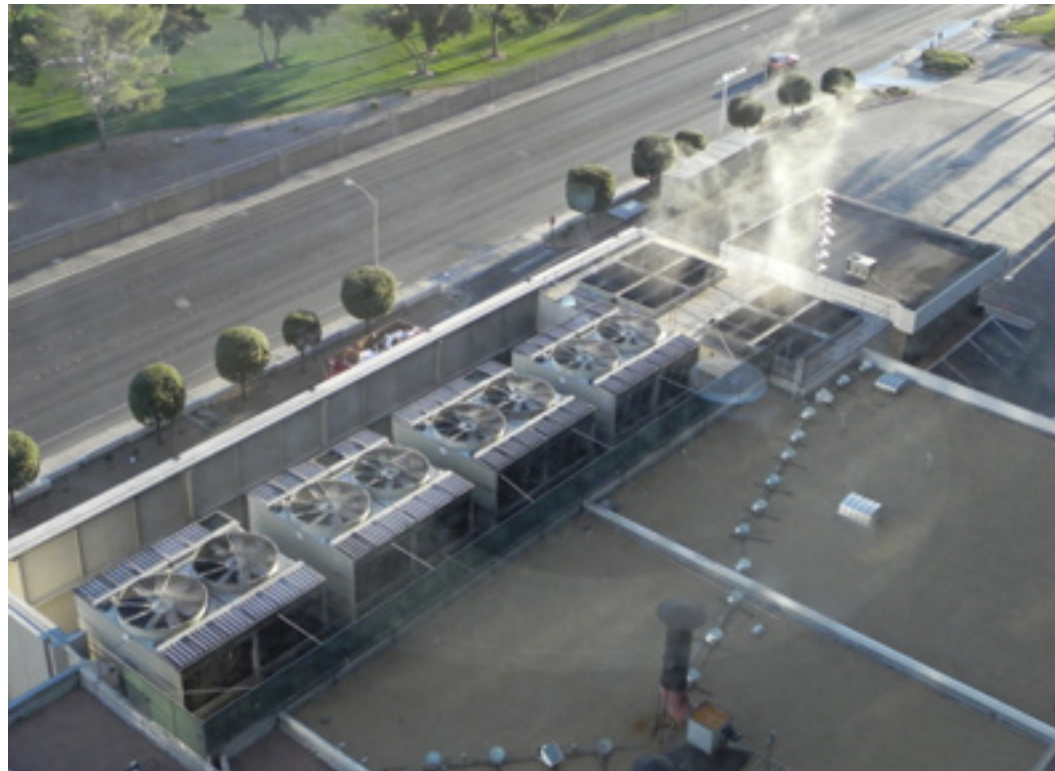
Cooling towers in operation with mist coming up from the cooling towers.
