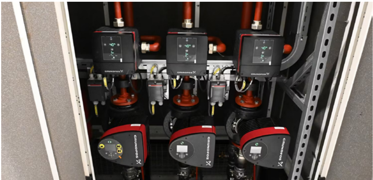
Figure 11 NorthC data centre intelligent flow-control installation
