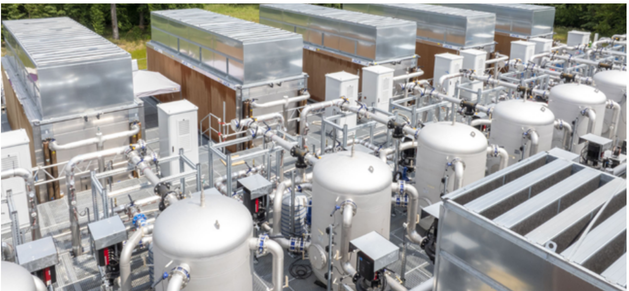
Figure 14 warm-water direct liquid-cooling system at the JUPITER supercomputing centre
