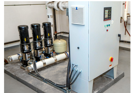
After Grundfos energy optimization upgrades
