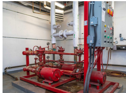
Original, oversized, inefficient pumping system
