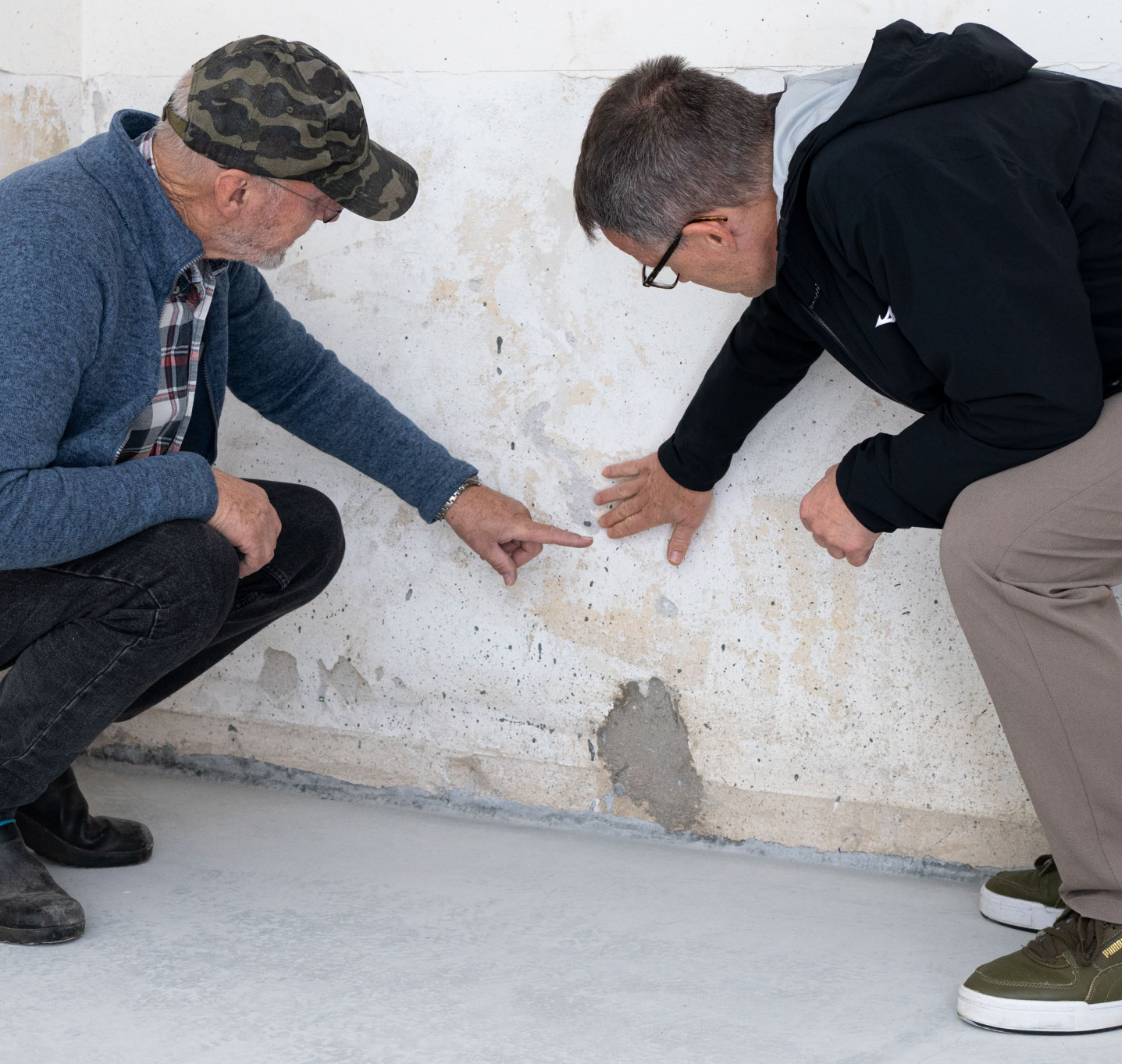
Homeowner John Sørensen and Global Product Specialist in Domestic Wastewater, Bjarni Rom-Jensen, inspect the basement walls for mold and cracks.
