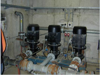
Fixed speed operation pump
