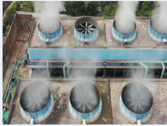
Uncontrolled fan operation
