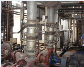
Valve control operation
