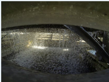
Uncontrolled water blowdown
