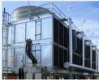
No dynamic control on cooling demand
