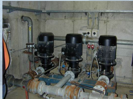
Industry wants to upgrade pumps
